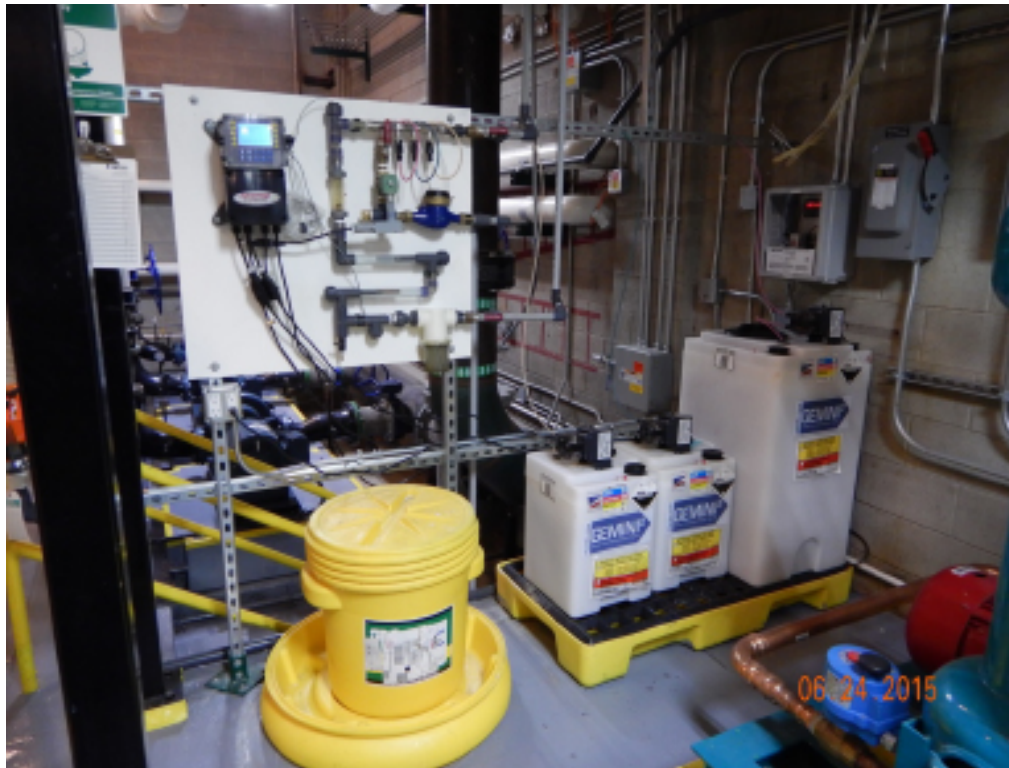
Figure 4. Chemical containers and side-stream filtration system used by the chemical scale-inhibition system
