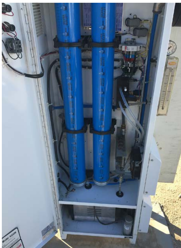
Figure 2. Inside of cabinet AOP technology Photo from Silver Bullet (now Clear Comfort)
